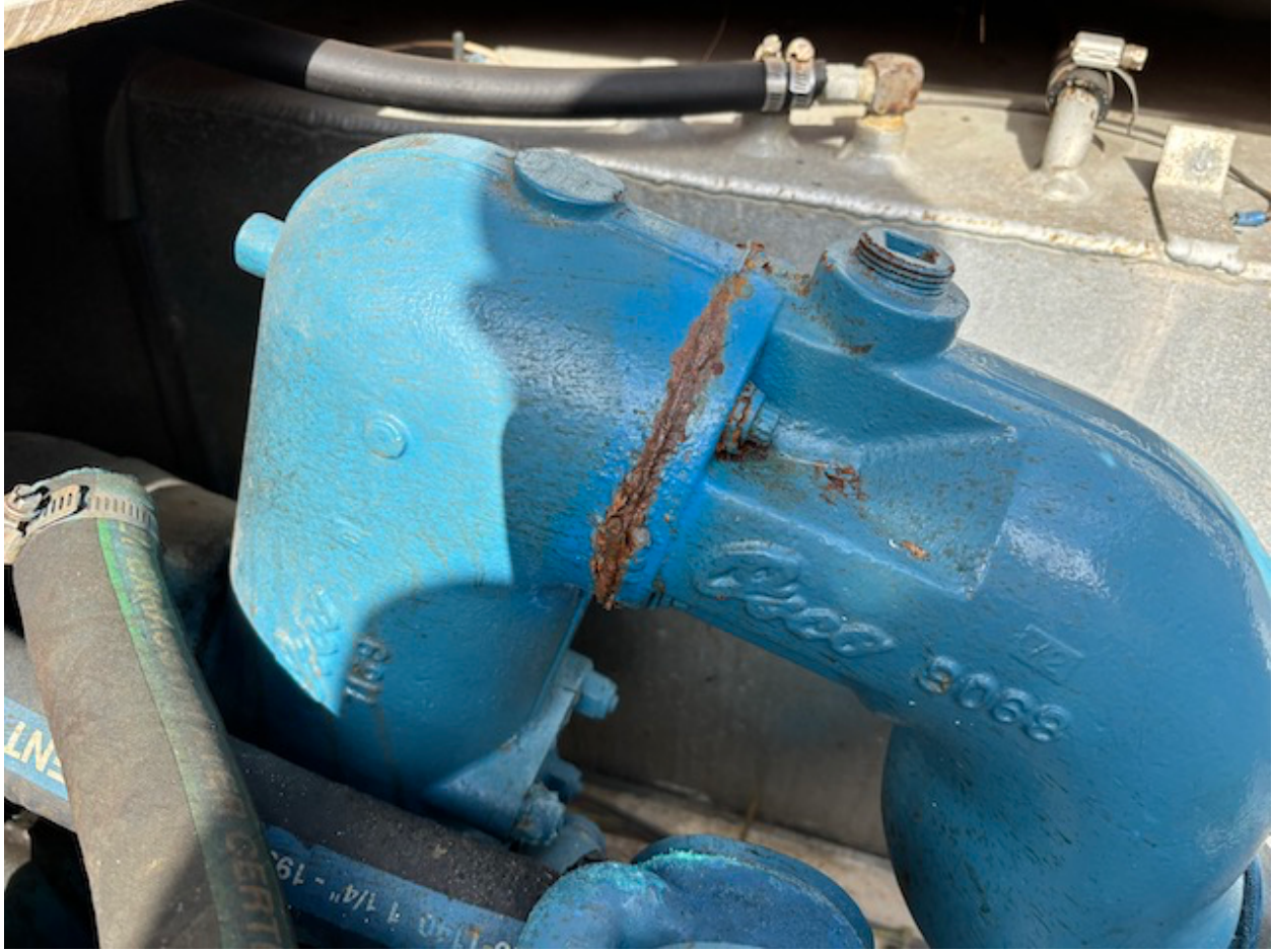
Starboard exhaust riser
