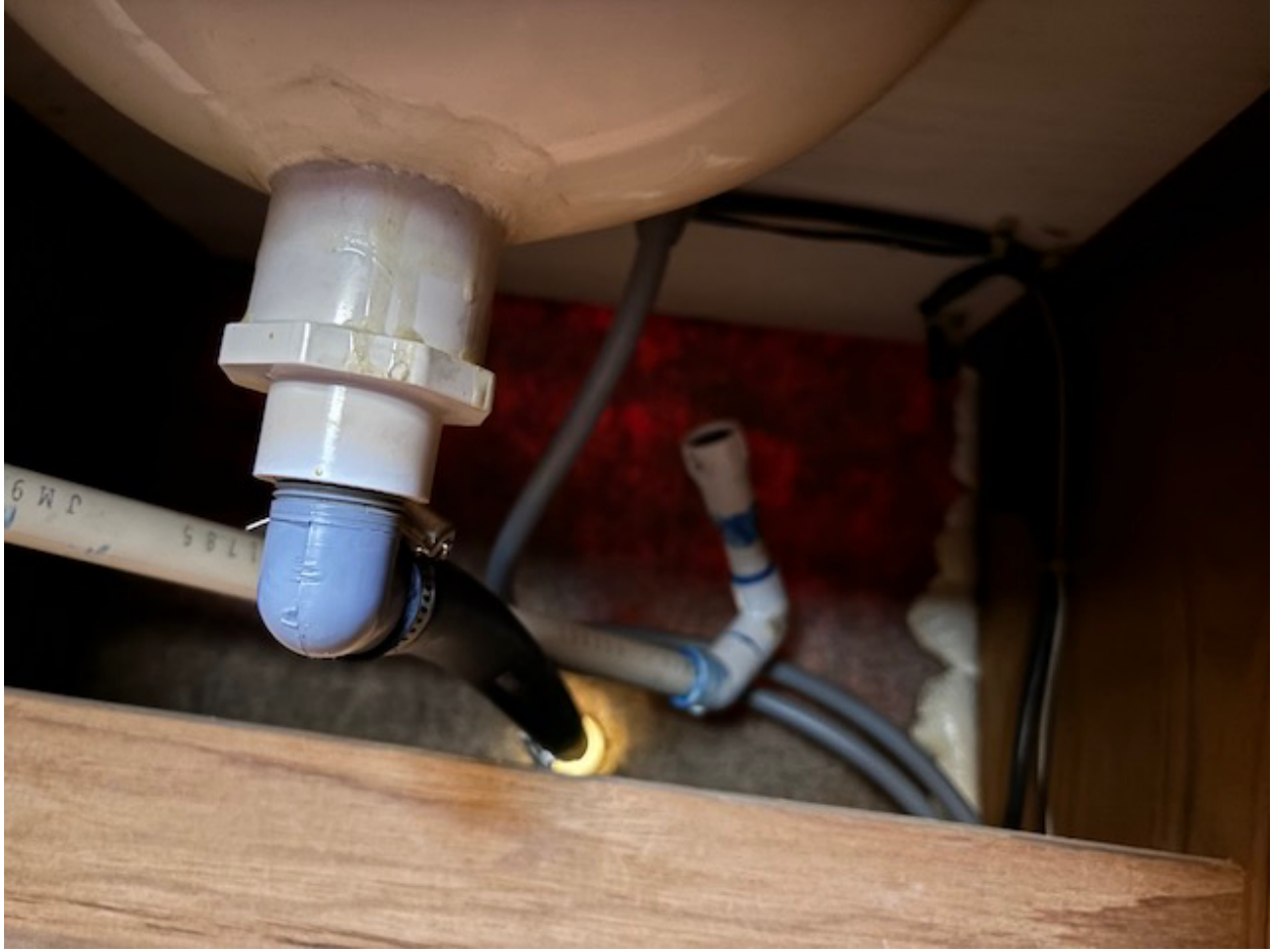
Under pilot berth sink
