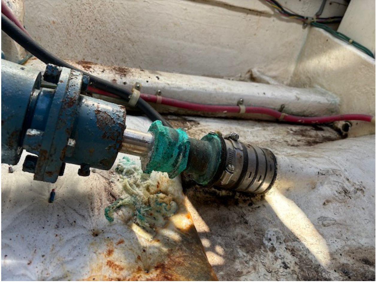
Starboard shaft seal.
