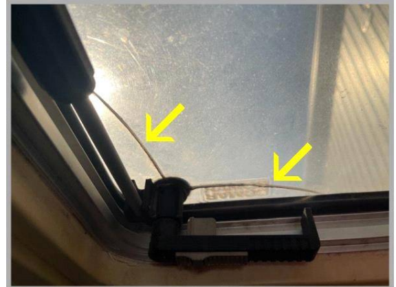
Cracked deck hatch
