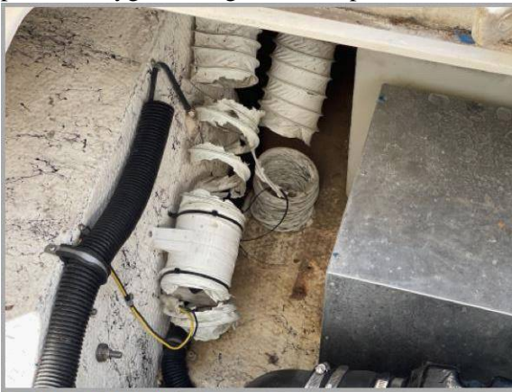
Engine ventilation hoses are torn
