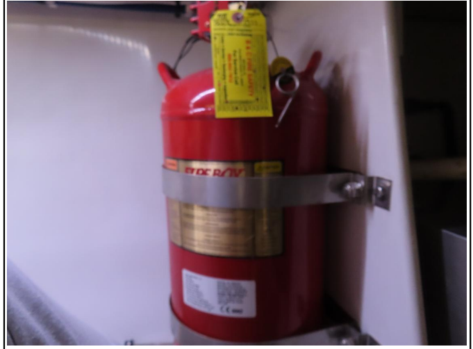
Engine room fire suppression
