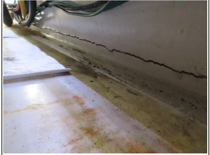
Starboard engine stringer crack
