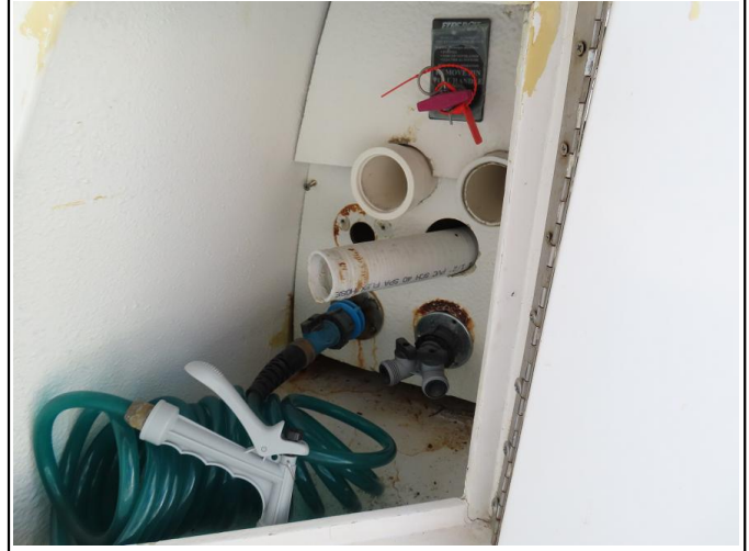
Cockpit water outlets
