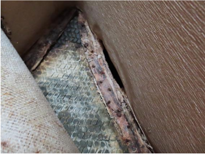
Bow cabin wood rot
