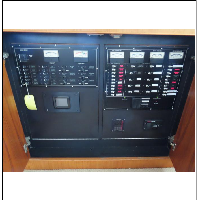
Salon breaker panel
