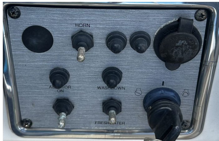
DC switches located at helm
